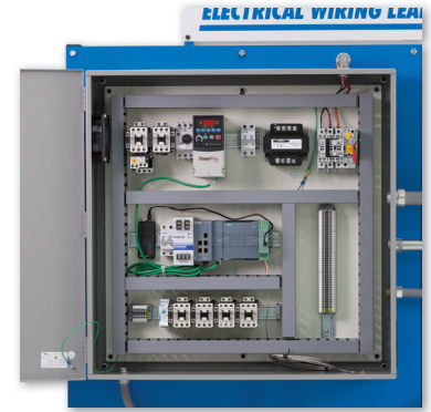
VFD & PLC Mounted in Panel
